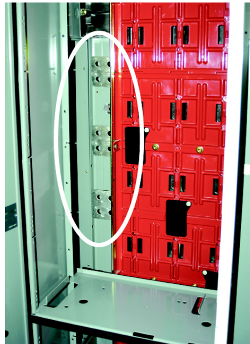
Bus Splice Access Cover Removed
