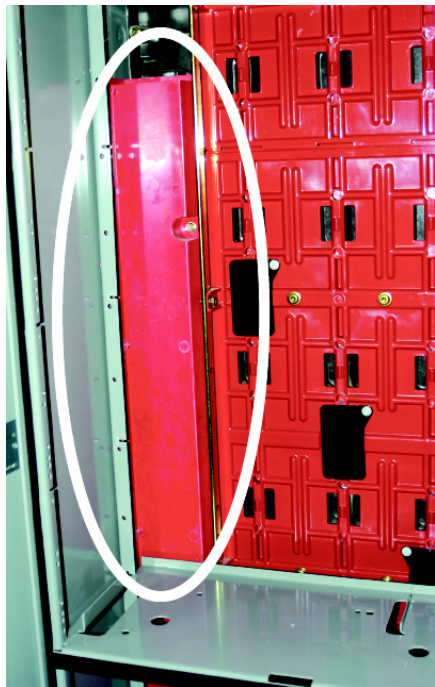
Bus Splice Access Cover In Place
