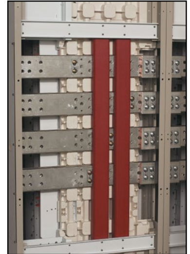
Rear view of main horizontal bus with covers removed
