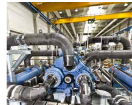
A compressor for nitrogen service
