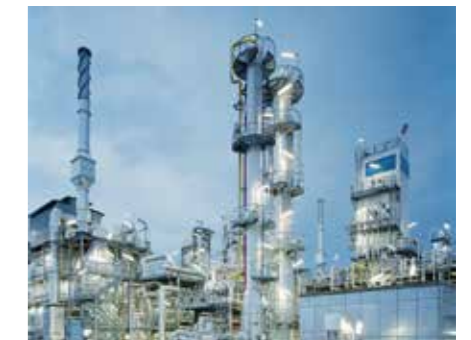
The growing HyCO market produces chemical feedstock gases and syngas. Photo: © Linde AG
