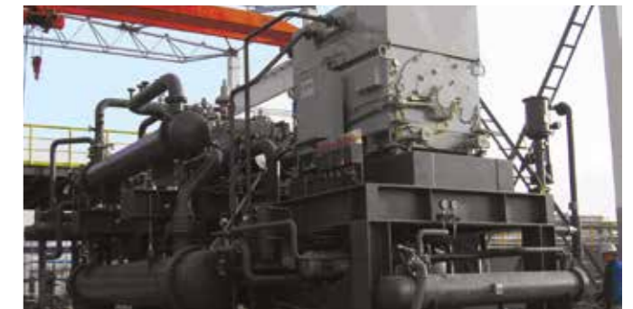
A centrifugal gas compressor for CO compression
