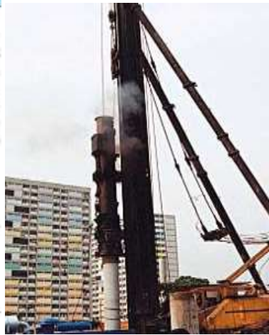
Underwater percussive piling strictly prohibited
