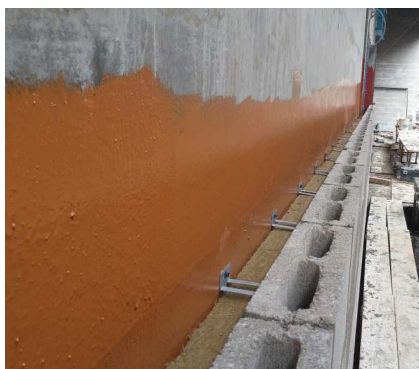
Fig. 1-5 Fluid-applied air barrier and WRB system field membrane over a concrete backup wall. Double eye and pintle masonry veneer ties penetrate through the exterior semi-rigid mineral fiber insulation.
