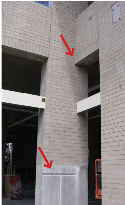
Fig. 1-20 Masonry veneer bears on concrete foundation elements below and loose lintel elements above openings as indicated
