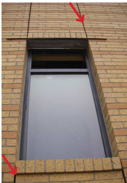
Fig. 1-18 Typical vertical brick expansion joint aligned with window jambs. Each joint continues the full height of the building and is awaiting backer rod and sealant joint installation.
