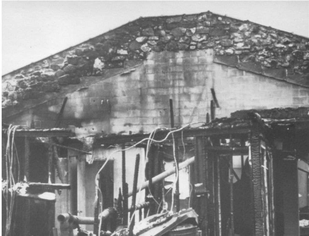
Figure 11.2.13. LWCMU Fire Wall Meets Expectations! Proven Performance in Actual Fires.
