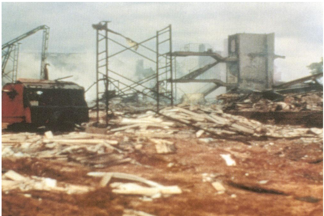
Figure 11.2.14. The only remaining assembly is the Elevator shaft constructed with lightweight Aggregate concrete masonry units.
