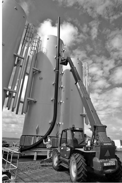
Figure 14: The J-tube through which the power cable is directed to the seabed.
