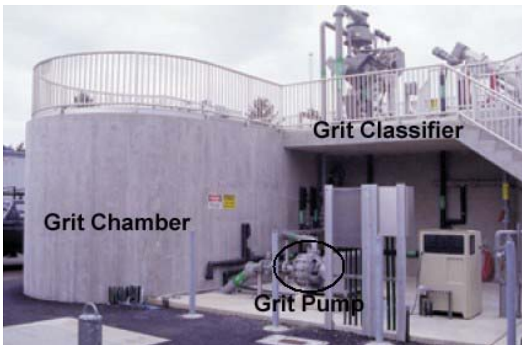
17 18 19 Figure 2.22 Photo of Pumps for Grit Removal 20 21
