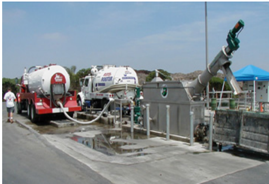
32 33 34 Figure 2.2 Septage Receiving Station
