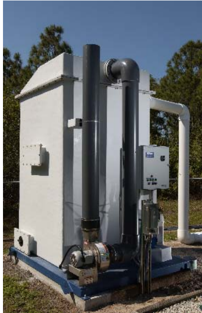
2 3 4 Figure 2.28 Photo of a Biological Odor Control System
