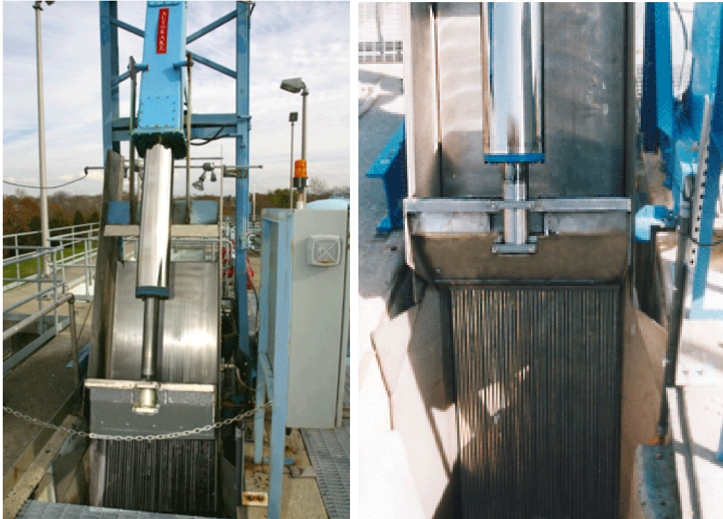
Figure 2.7 Front-Cleaning Mechanically-Cleaned Bar Screen
