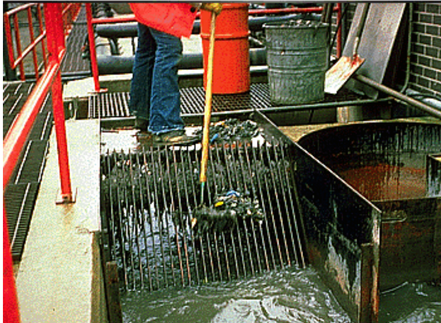
9 10 11 Figure 2.5 Manually-Cleaned Bar Screen 12
