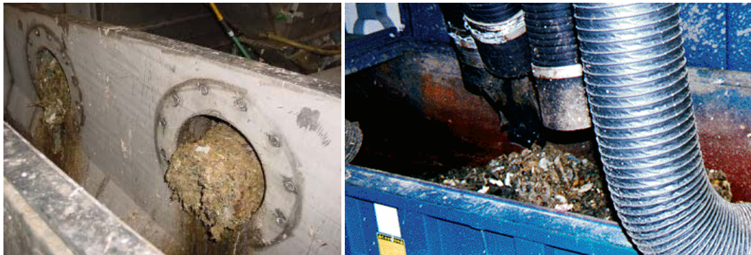
Figure 2.15 Screenings Being Collected
