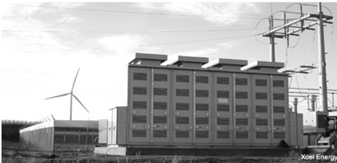
Figure 9: 6 MW, 8 h Sodium-sulphur energy storage facility in Tokyo, Japan [2].
