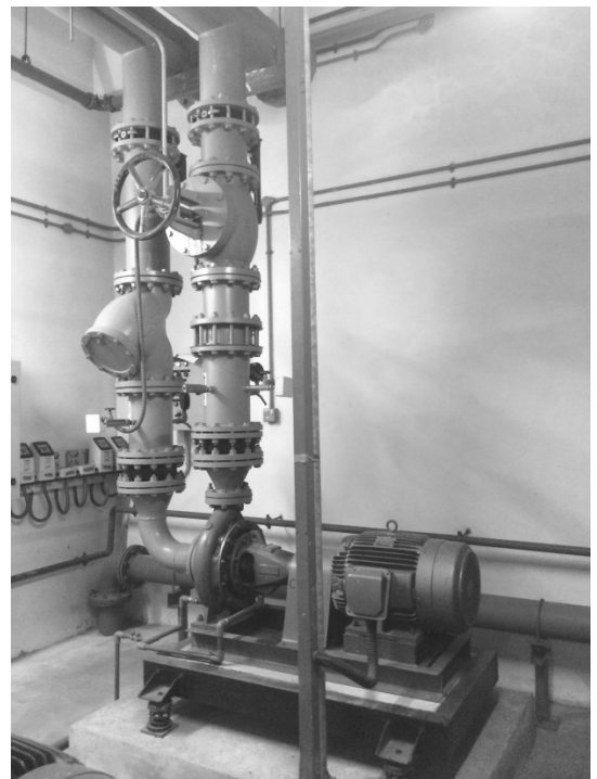
ပုံ ၆-၉ Condenser water pump pipe connection
