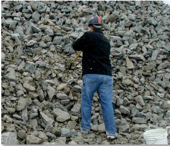
Photograph 8-19. Seven-inch minus crushed surge is a key ingredient to fill gaps between riprap.
