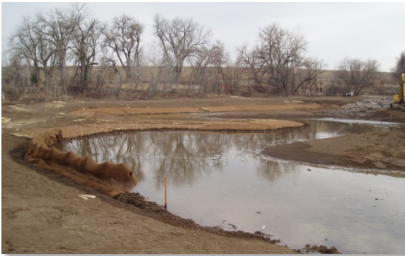
Photograph 8-13. Coir blanket used to protect the outside banks of a low-flow channel immediately following construction.
