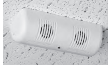
Figure 9.12.8. Ceiling occupancy sensor.
