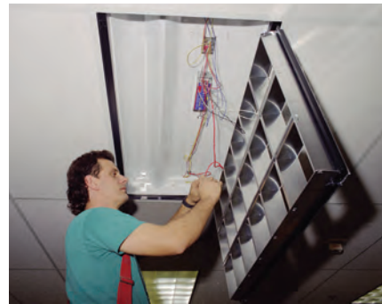
Figure 9.12.4. Repair and rewiring must be done by a licensed electrician.
