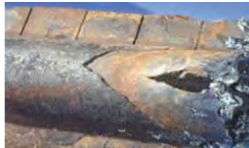
Figure 9.2.9. Boiler tube – failure (rupture)
