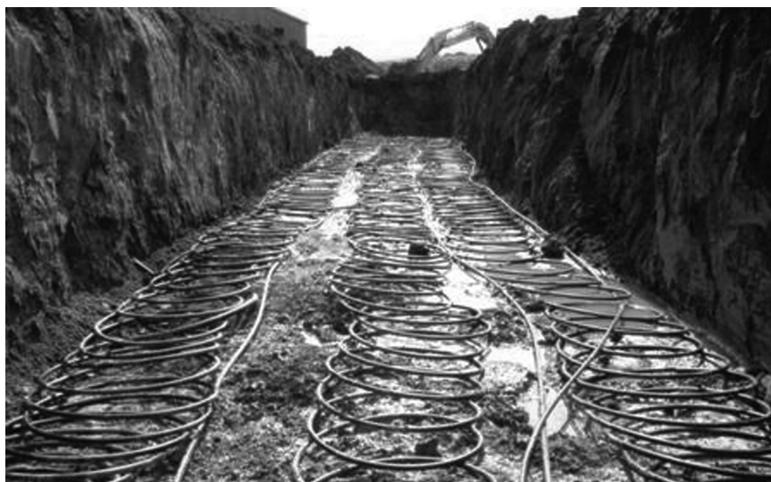
Figure 6.11 A horizontal closed loop field is composed of pipes that run horizontally in the ground below the frost line—photo shows a “slinky” (overlapping coils) arrangement before it has been covered by dirt. The slinky style layout is a more space-efficient version of a horizontal ground loop than straight piping. (Image by Marktj released to the public domain; http://en.wikipedia.org/wiki/Geothermal_heat_pump )
