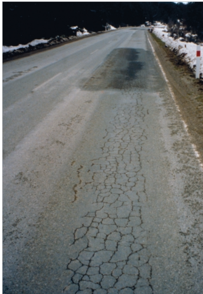
Figure 3-30 Alligator cracking has a cracking pattern like an alligator skin.
