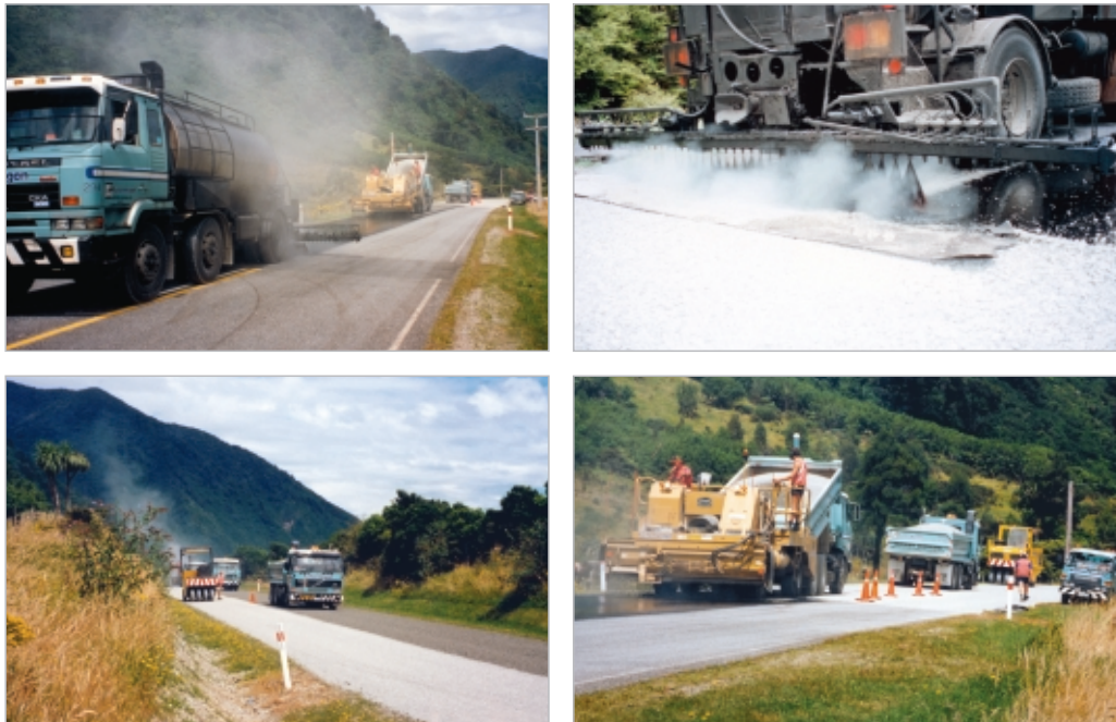
Figure 3-7 Constructing a chipseal. Clockwise from top left: Spraying binder and spreading chips in one operation. Top right: Spraying the binder. Bottom right: Spreading the chips. Bottom left: Rolling the surface. Photos courtesy of Les McKenzie, Opus
