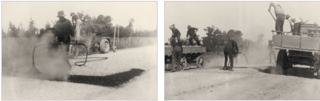
Figure 3-6 Constructing a first coat chipseal near Gisborne in the 1920s was not highly mechanised, compared to the line of construction machines used in the 2000s shown in Figure 3-7. Left: Hand spraying the basecourse, from the tractor-drawn bitumen distributor. Right: Spreading the chip by shovel as the tip truck was not yet in use. Photos courtesy of John Matthews, Technix Group Ltd
