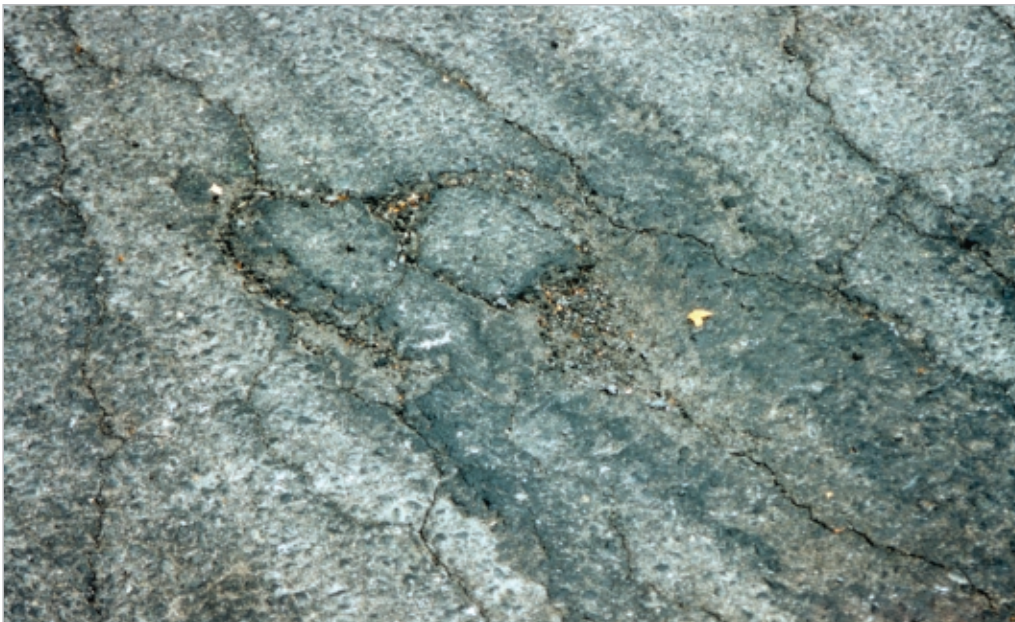
Figure 3-33 Potholes and cracks form where water gets under the pavement.
