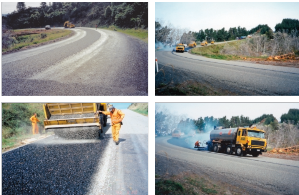
Figure 3-16 A sandwich seal under construction in Hawke's Bay. Clockwise from top left: Applying the first layer of large chip to the flushed surface without binder. Top right: Applying the binder over the large chip. Bottom right: Applying the binder over the large chip. Bottom left: Small chip being spread over binder over large chip.
