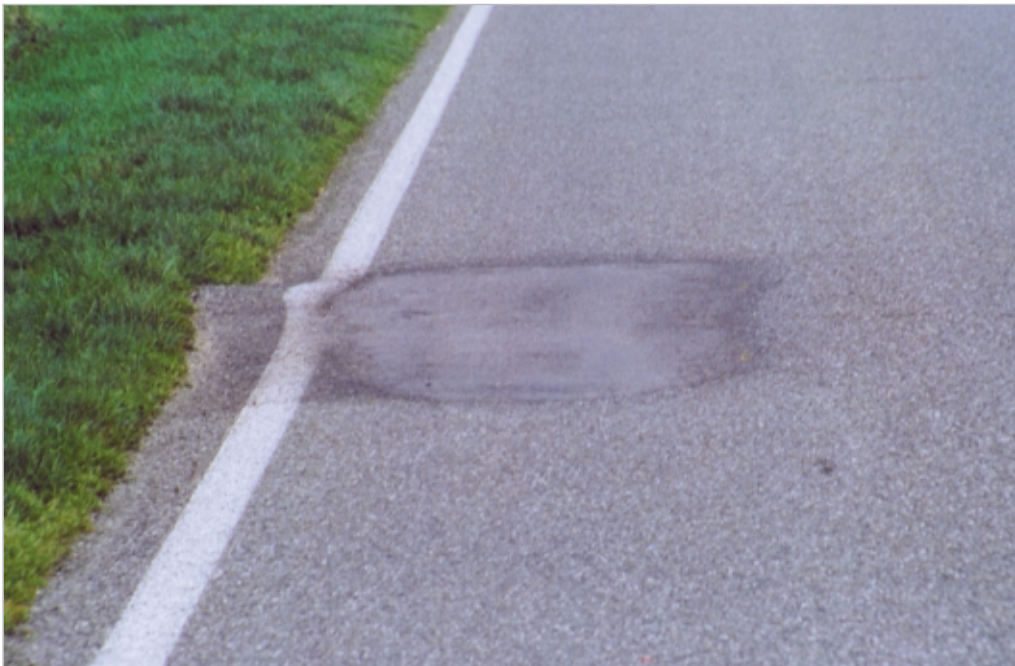
Figure 3-28 Shoving in a pavement.
