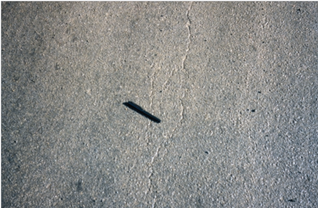
Figure 3-31 Longitudinal and transverse cracks run along or across the road.
