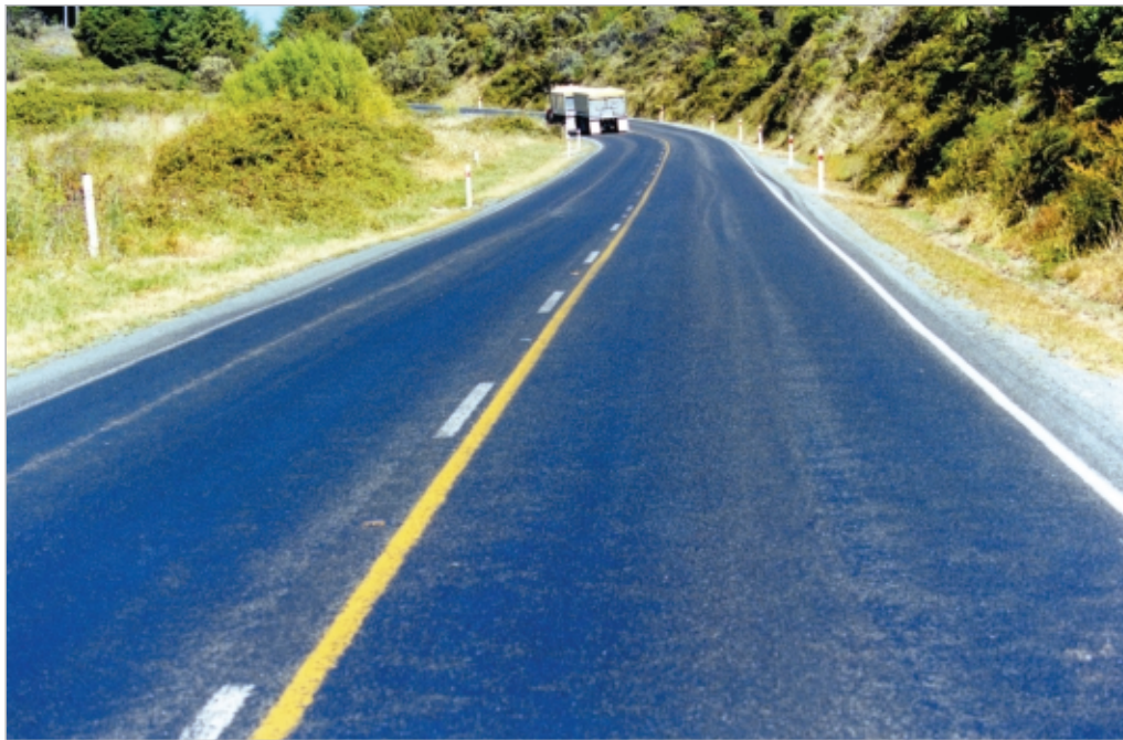
Figure 3-35 This road shows a slick, bleeding or flushed surface that has low friction and therefore low skid resistance. Photo courtesy of Mark Owen, Transit NZ
