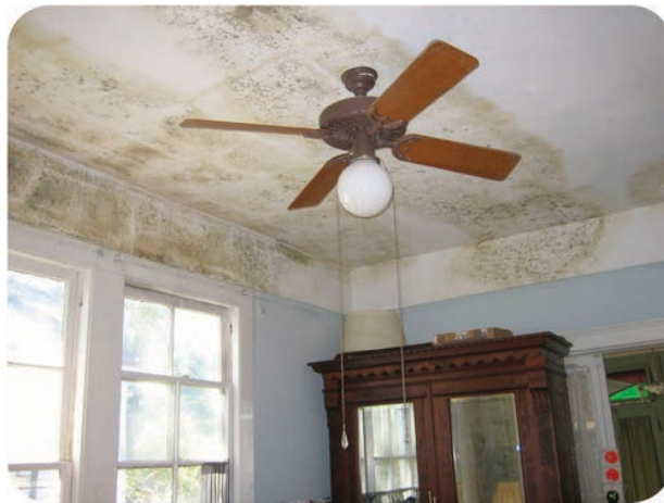
The mold growing on the walls and ceiling of this storm-damaged home may be harmful to human health.
