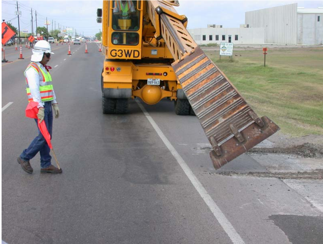
Figure B3. Pavement Excavation along the Shoulder at the Vicinity of the WIM Site.
