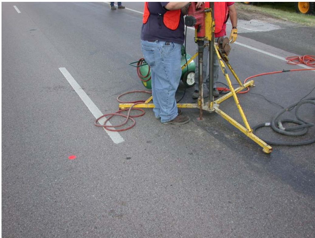
Figure B2. Drill Mounted on a Tripod to Drill a Hole for the MDD.
