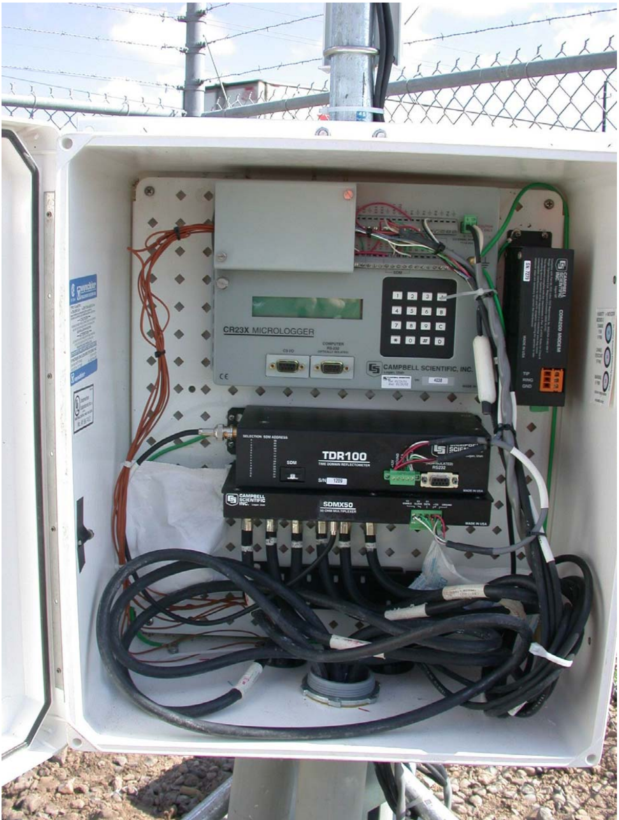
Figure B15. Weather Station Controller Box.
