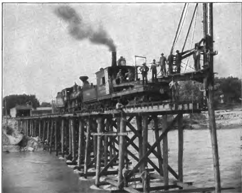
B. PILE DRIVER CONSTRUCTING TEMPORARY BRIDGE OVER NEW NORTH CHANNEL, LAWRENCE, KANS.
