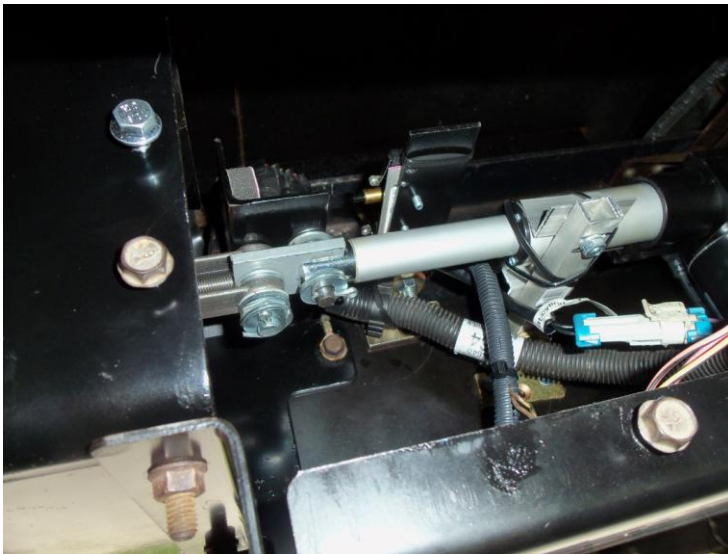
The installed park brake unit with the actuator extended (brake off).
