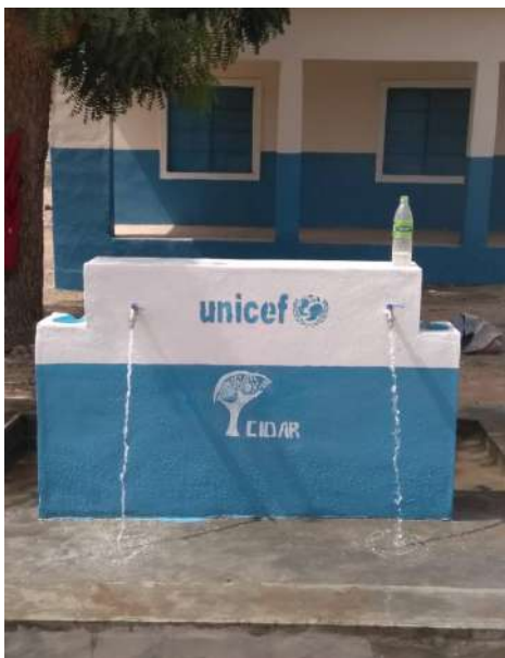
Picture 13: Handwashing Station in GSSS Banki, Bama LGA
