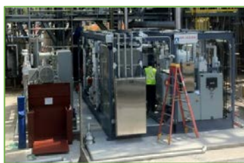
Cold Membrane System (American Air Liquide, Inc.)
