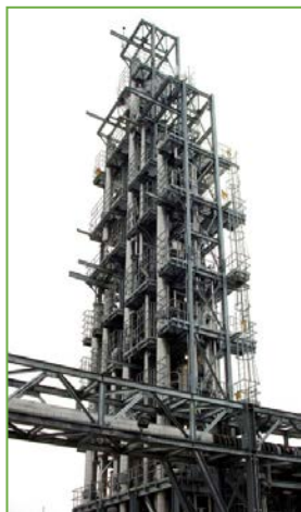
NCCC: 0.5 MW PSTU, 1 MW test bay (CCSI/Cansolv)
