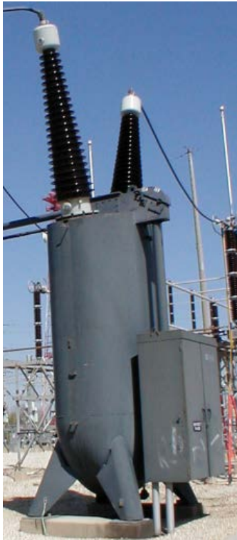
Dead tank breaker
