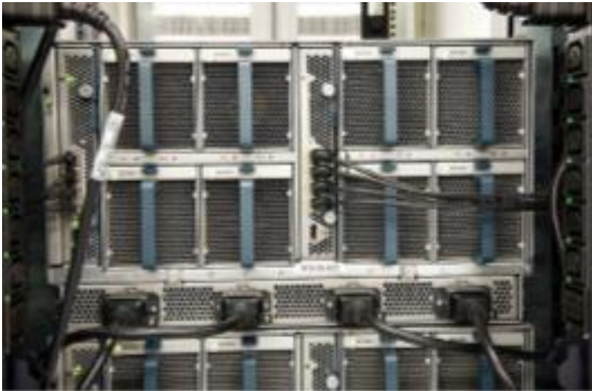
Cisco Unified Computing System
