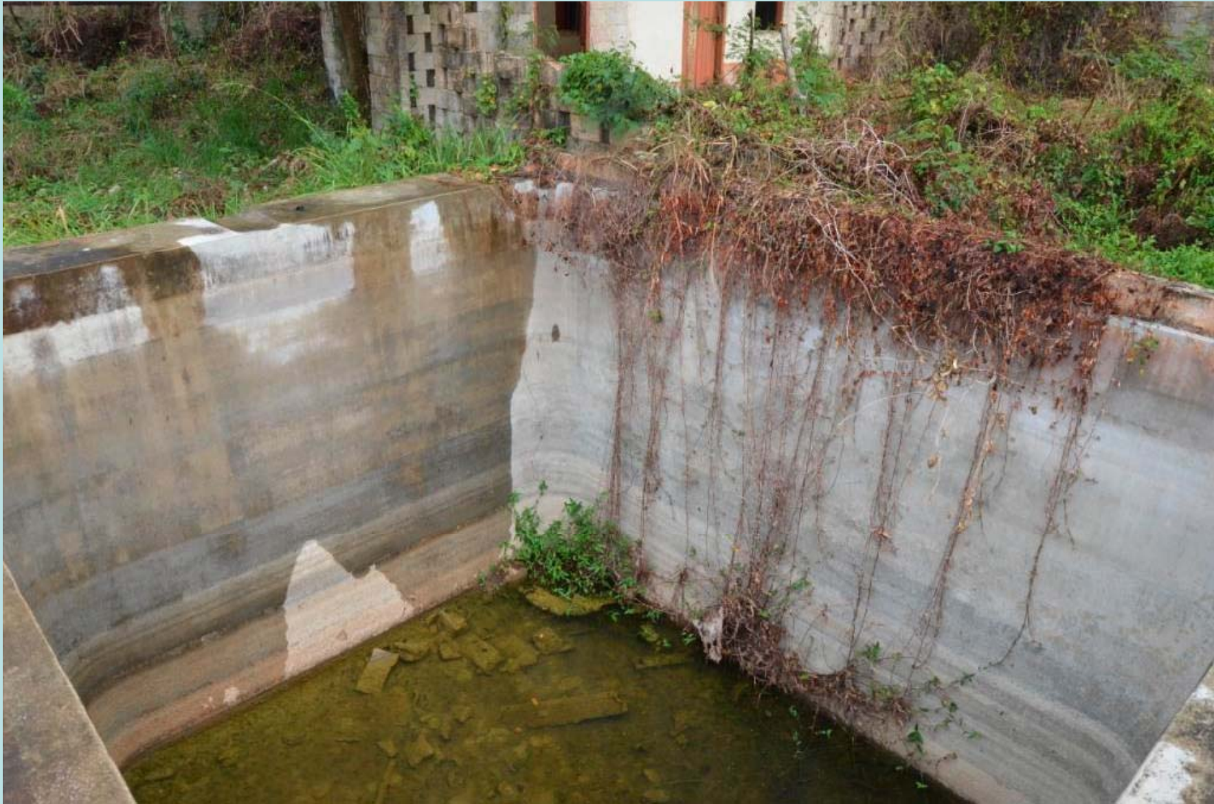
The depth and interior construction of a cistern. This cistern is about 12 feet in depth. Southfield, Jamaica
