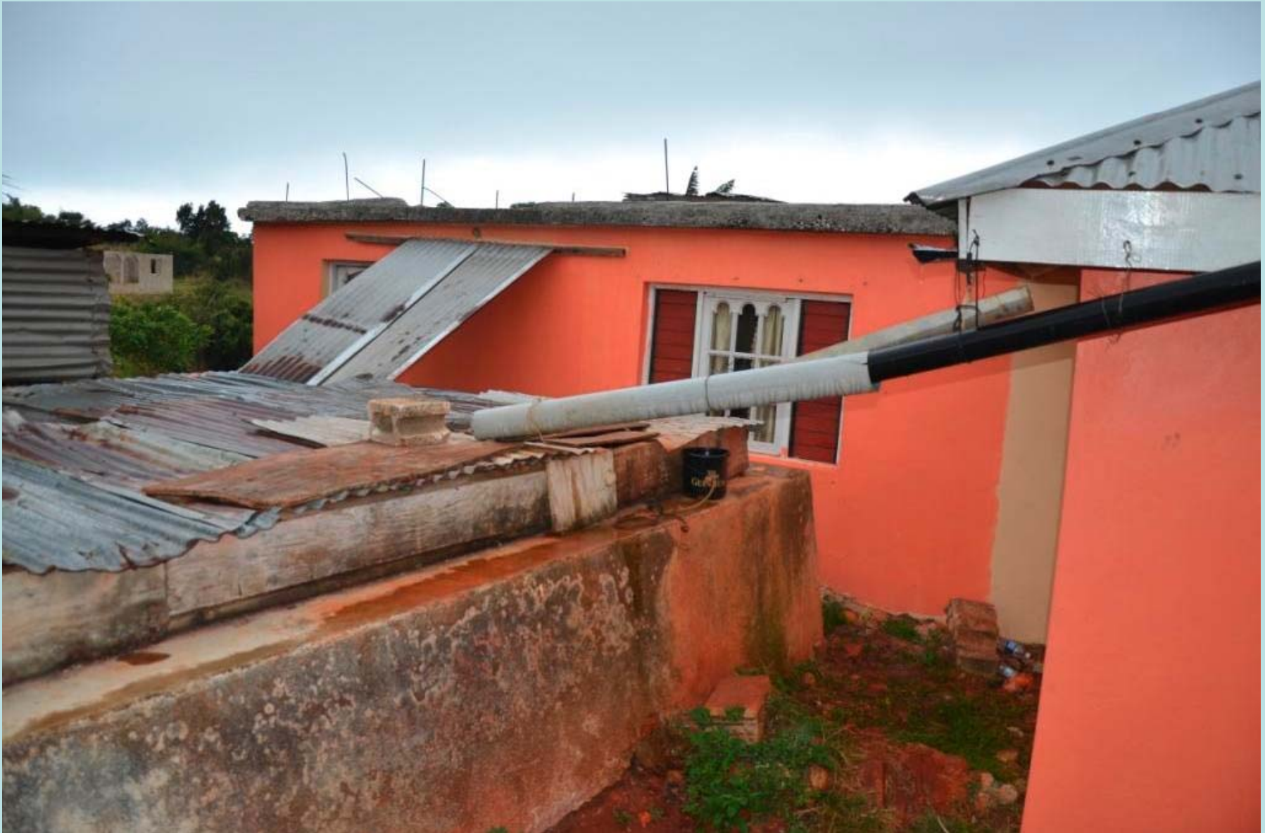
Water moves into the cistern from both roofs of the house, and directly through the slats of the metal roof covering the cistern. This area usually gets about 38" of rainfall a year. House A, Queensbury, Jamaica
