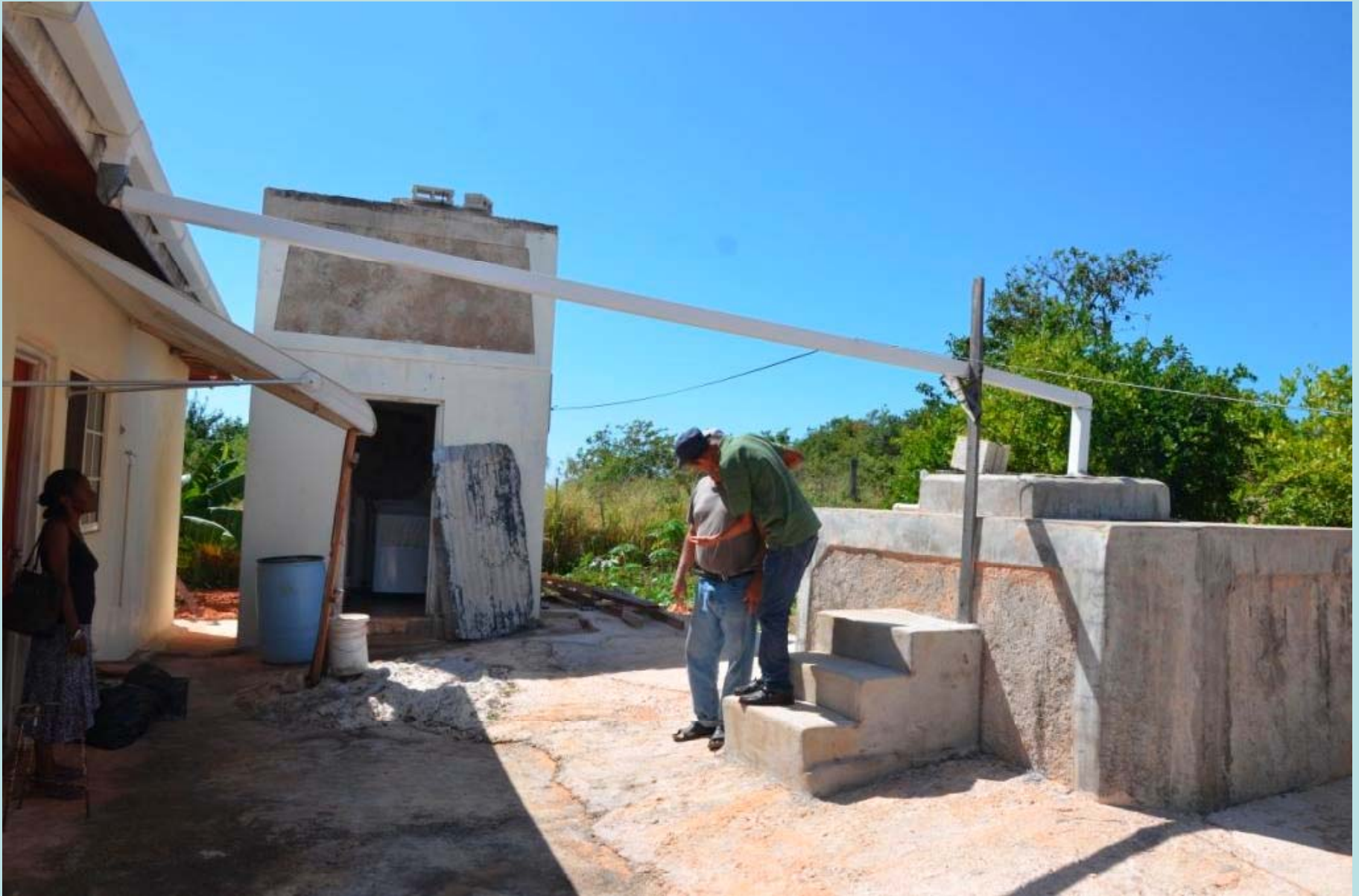
Here, water is collected into the cistern from the roof and pumped upwards into the air tank (center) and gravity fed into the house. The bottom of the air tank serves as the laundry room and supplies water to the washing machine.
