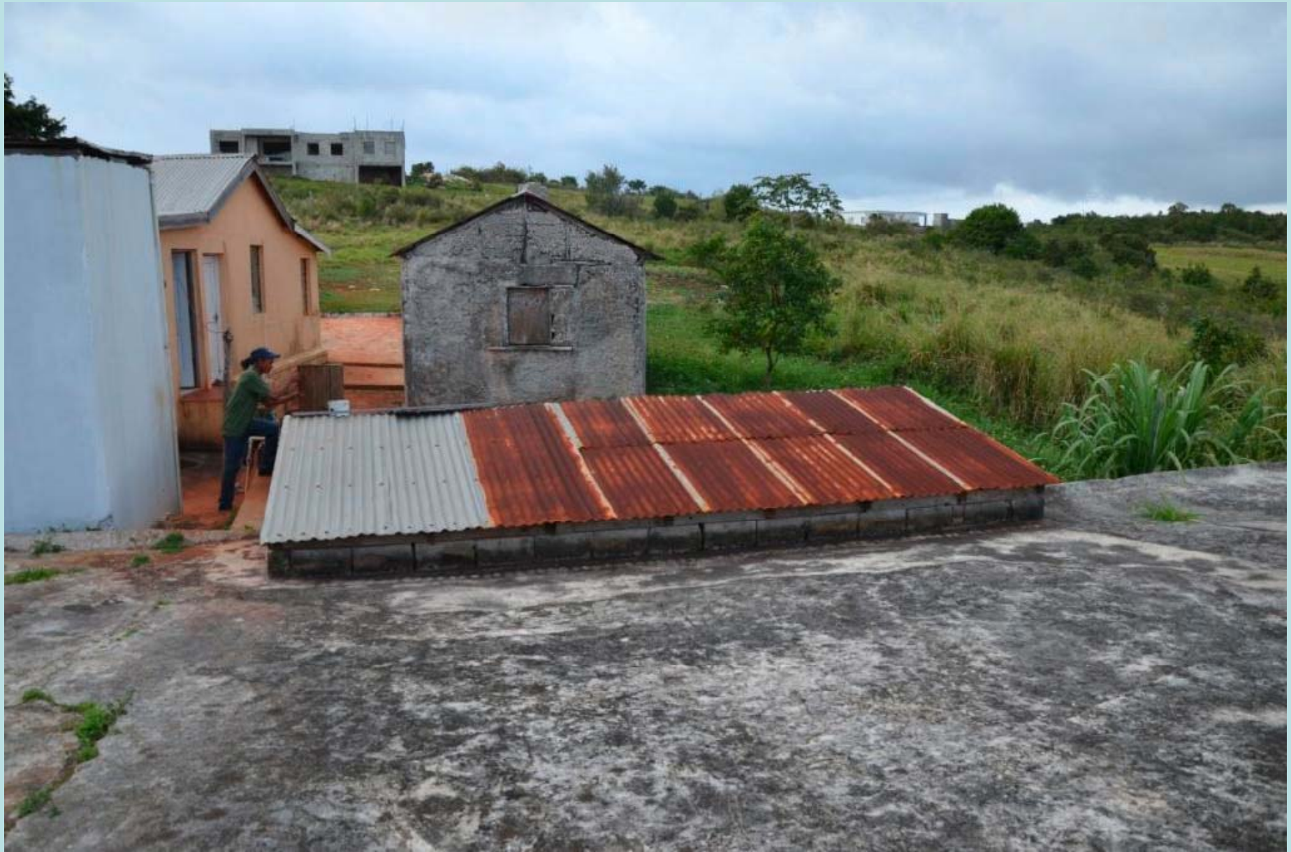
In this case, water flows from the sloped concrete slab in the foreground, which is also part of the cistern, and into the lower portion of the cistern having the metallic roof. House B, Queensbury, Jamaica
