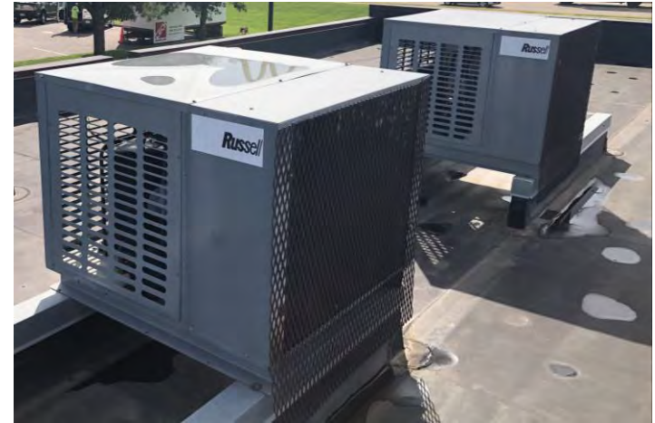
Condensing units – Liquor Store
