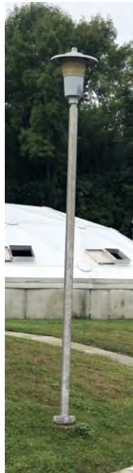
HID exterior lighting at WWTF - Typical
