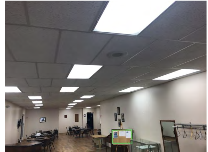
Senior Center Fluorescent Lighting
