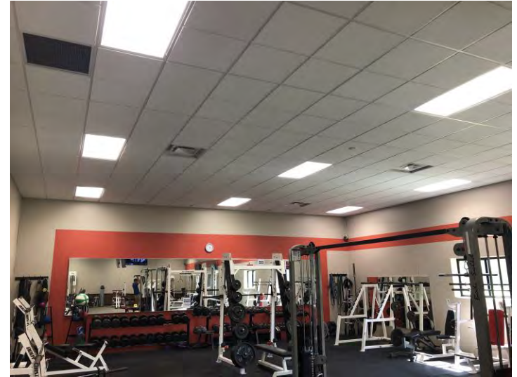
Fitness Center fluorescent lighting
