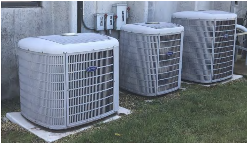
Condensing Units – Police Station
