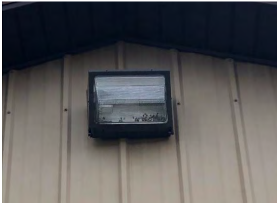
High Pressure Sodium Wall-Pack at Park Garage - Typical
