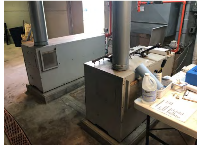
Existing Boilers - Pool
