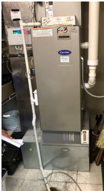
Furnace – Police Station
