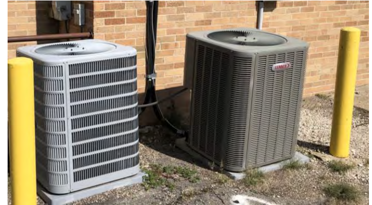
Condensing Units – City Hall
