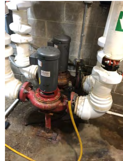
Pumps – Crescent Apartments
