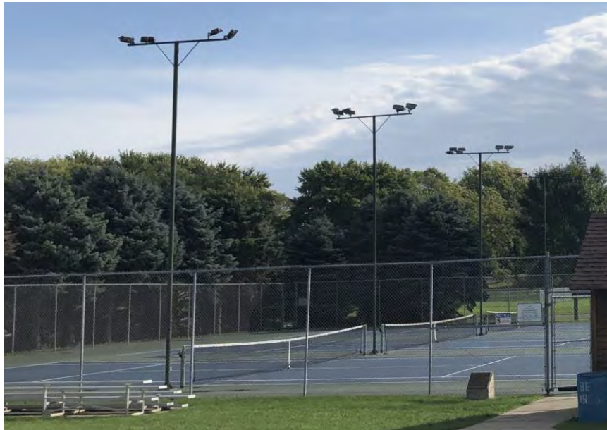
Existing Flood Lights – Tennis Courts
