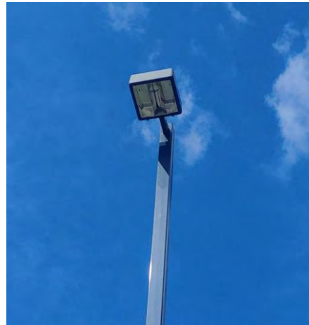
LED Installed in Old HPS Shoebox Fixture
