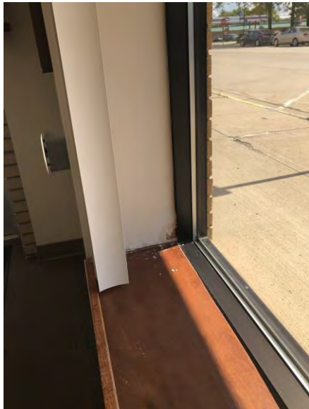
Leaking Window Frames – Library & Senior Center
