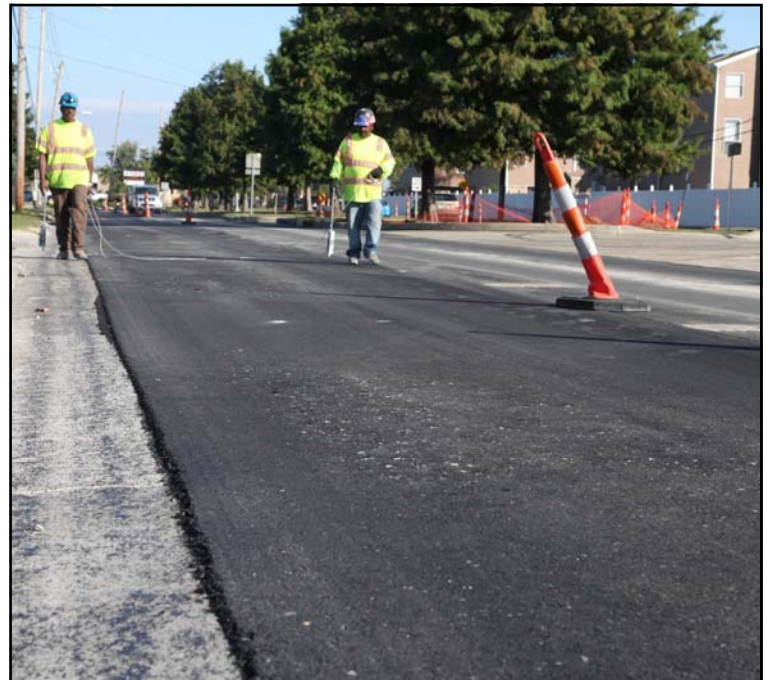
Resurfacing along West Esplanade in Kenner is part of the Paths to Progress program, a joint venture between State and Federal agencies resulting in approximately $26 million being spent on Kenner roadways.
