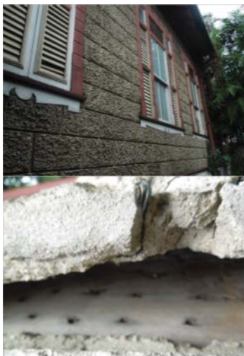
Figure 13: Side façade of the Boissière House: In this photo some of the plasterwork is removed to show the use of nogging below Source: Photo taken by the author, Jan 2010 Source: Photo taken by the author, Jan 2010
