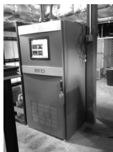
New KUSC 13,000 watt digital FM transmitter installed and running.
