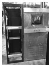
New KUSC Transmitter just after delivery, still wrapped in plastic.
