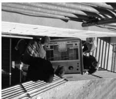
Delivery of new transmitter to KUSC mountain top building in Angeles Forest
