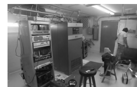
KDB Transmitter Room at Gibraltar Peak/ Move in and Clean Up
