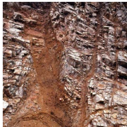
Figure 43: Weakness (crushed) zone. A central core of sand/clay, filled joints (shears?) branch out. A borehole along the zone will give completely different results compared to a borehole across the zone.
