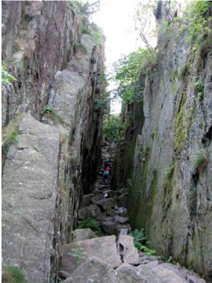
Figures 22: Weakness zones in the surface. Eroded weakness zone/fault
