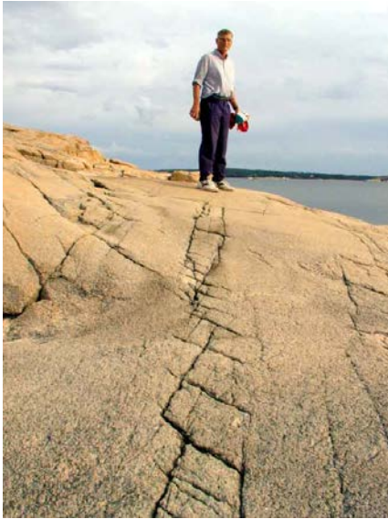
Figure 18: Very short joints in a granite.
