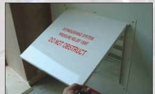
Figure 9: The sign says "DO NOT OBSTRUCT" because it is very likely the vent path will be obstructed, thus the vent path must be checked regularly.
