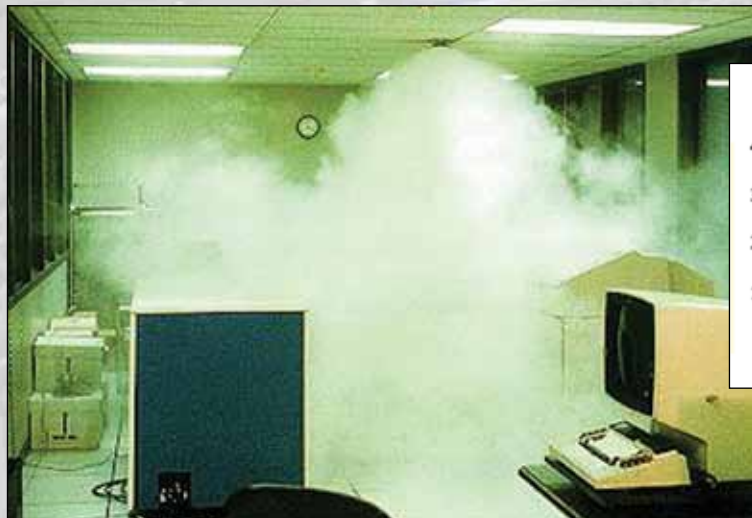
Figure 1: The clean agent expands, causing cooling which condenses moisture to form a fog.
