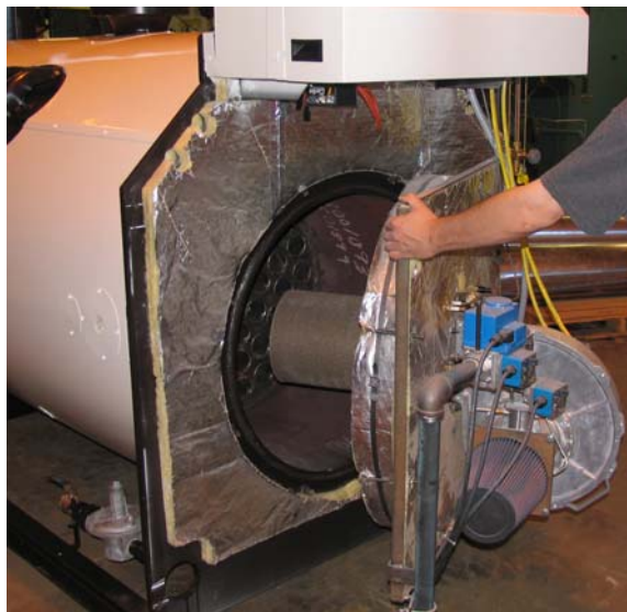
Figure B6-4. Burner maintenance
