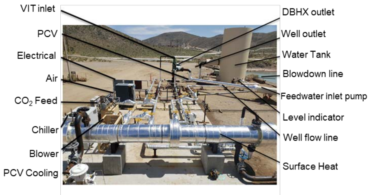
Figure 6: Surface Equipment Layout
