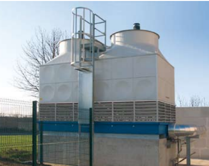
Cooling tower type CMC 2.9 Chemical Plant in France
