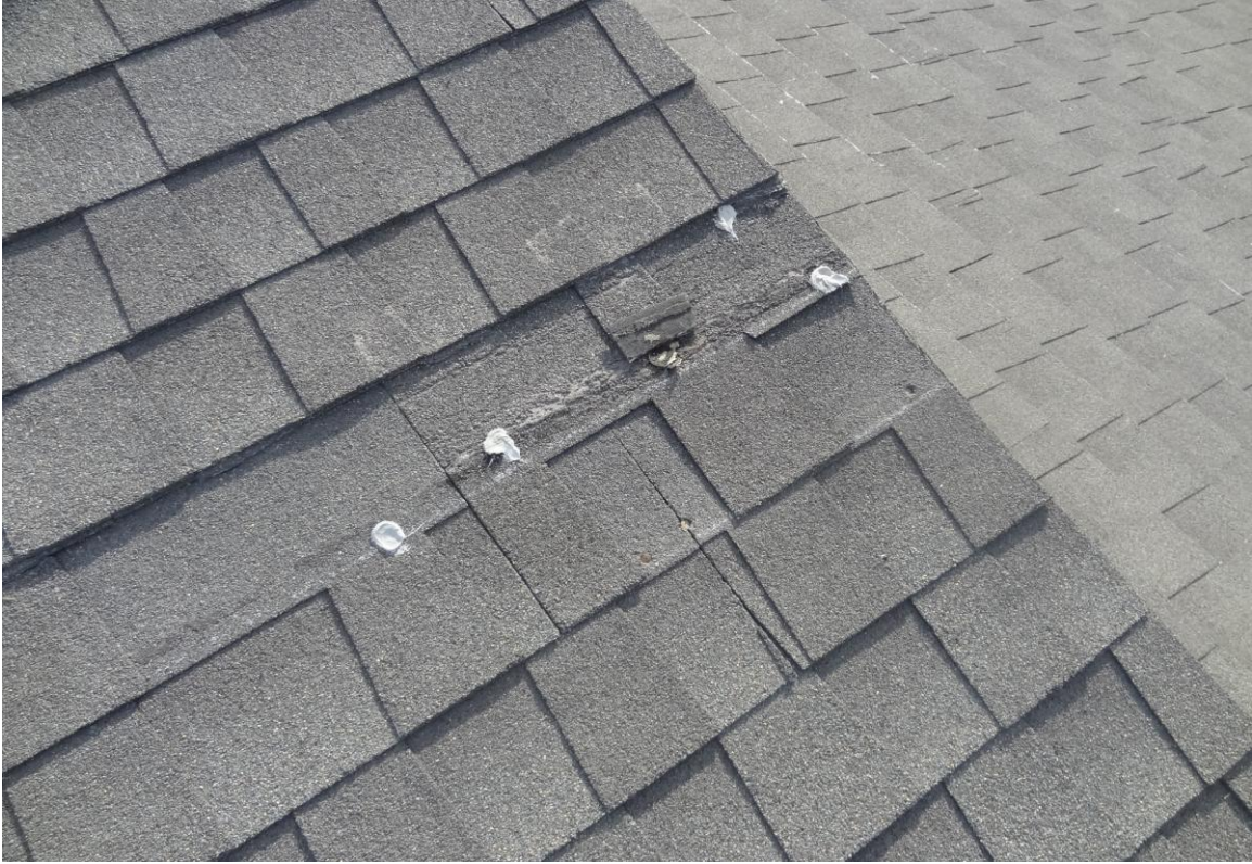
NDF / State Parks Office Building – FCA Building #2033 Description: Damaged shingles.
