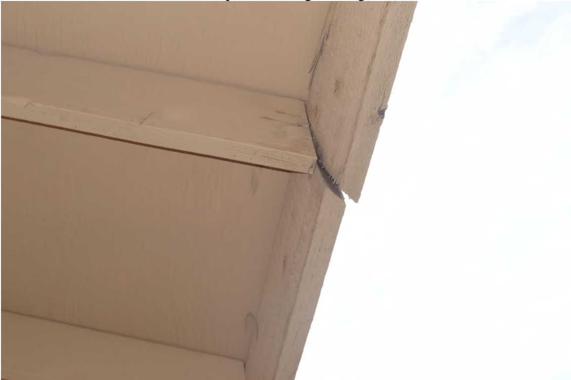
NDF / State Parks Office Building – FCA Building #2033 Description: Damaged fascia board.
