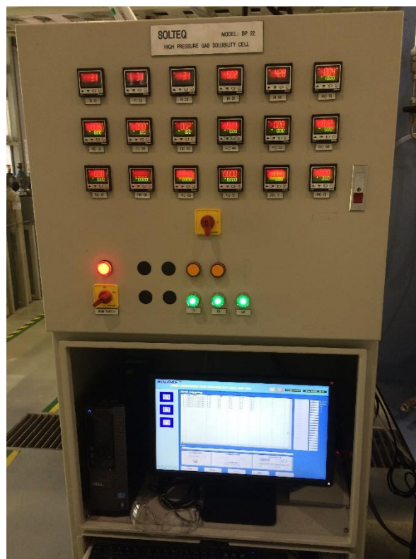
FIGURE 7 Main control unit
