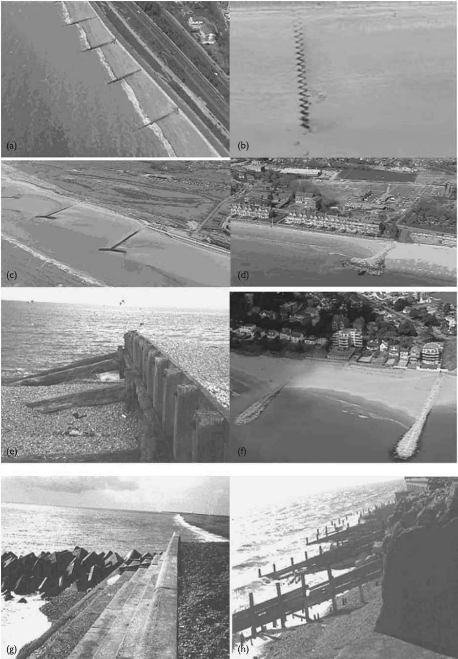
Figure 9.3 Groynes (a) typical groyne field; (b) zig-zag groynes; (c) 'T' head timber groynes; (d) 'T' head rock groyne; (e) massive timber groynes; (f) rock groynes; (g) concrete armour terminal groyne; (h) timber piled (deteriorated).
