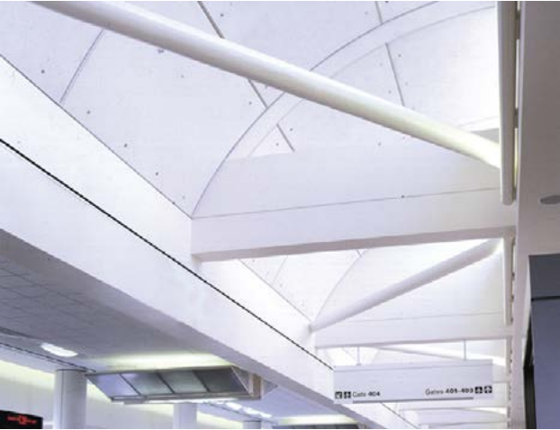
The proper thickness of the intumescent coating is critical for providing the required fire rating.
