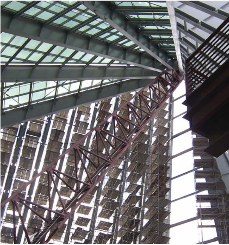
A high-performance polyurethane coating based on polyaspartic ester technology was applied to the steel beams of the National Museum of the Marine Corps, Quantico, VA. Photo courtesy of The Sherwin-Williams Company.
