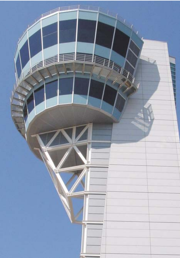
A solvent-borne vinyl mastic intumescent coating was applied to the exterior structural steel of this air traffic control tower.
