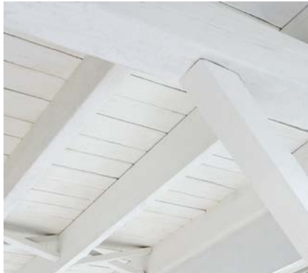
Fire-protective materials are often specified in existing buildings where adaptation or renovation for a new or different use is planned. Above: intumescent fire-resistive coating applied to a wooden floor/ceiling assembly as part of a restoration program in an historic building.
