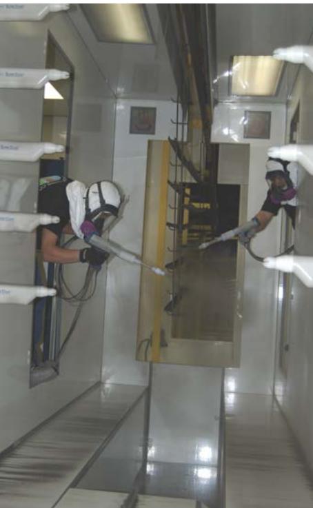
Application of powder coating to aluminum trim. Photo courtesy of Quality Powder Coatings LP.
