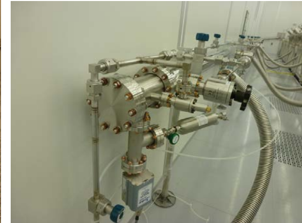
Swagelok backfill/purge start valves
