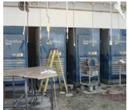
DWS on Granite Finishing 22,000 cfm (37,370 m 3 /h)
