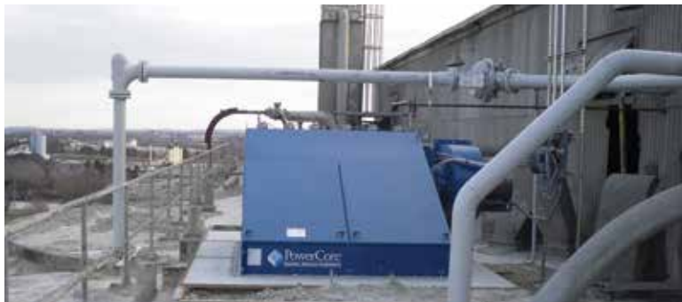
CPV - Multiple Cement Silos 4,800 cfm (8,154 m 3 /h)
