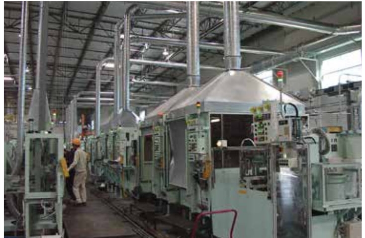
DFO on Welding Fumes 53,000 cfm (90,028 m 3 /h) Left: outside Right: inside
