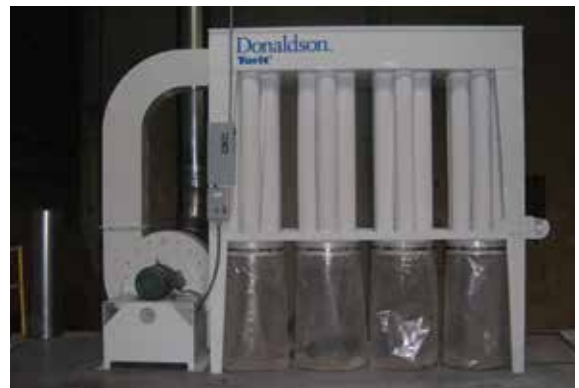
IRD - Wood Shop 5,000 cfm (8,493 m 3 /h)
