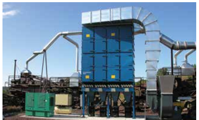
DLMC on Rock Crushing 41,000 cfm (69,645 m 3 /h)
