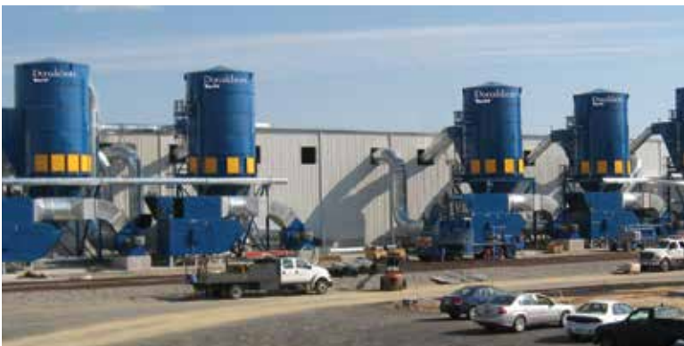
RF - Wood Furniture Facility 403,000 cfm (684,556 m 3 /h)
