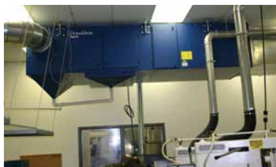
MODULAR MEDIAFILTER™ on Grinding 2,000 cfm (3,397 m 3 /h)
