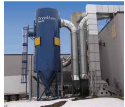
RF - Cabinet Shop 48,500 cfm (82,385 m 3 /h)
