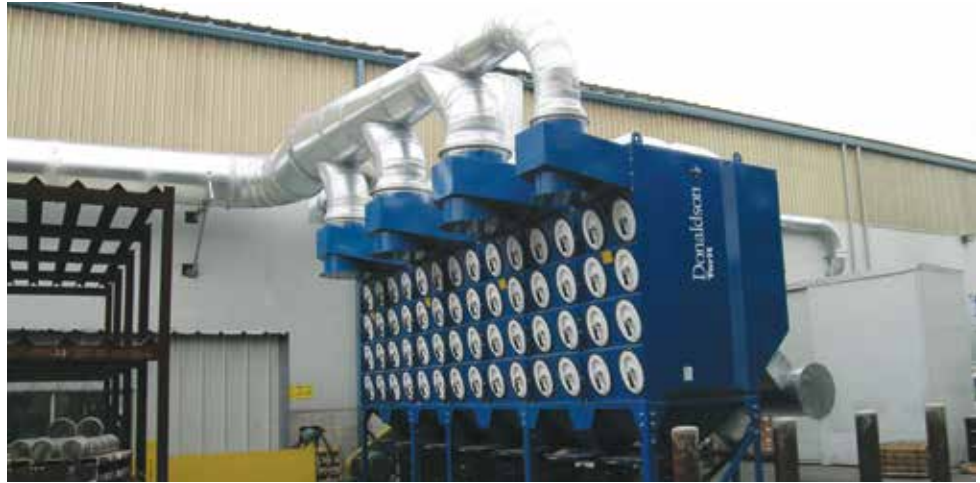
DFO on Grinding 74,000 cfm (125,700 m 3 /h)
