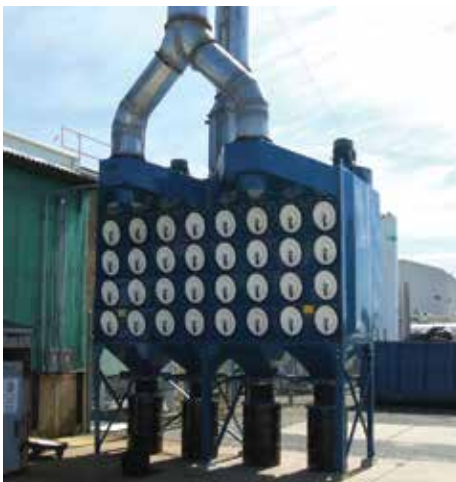
DFO on Thermal Spray 8,500 cfm (14,439 m 3 /h)
