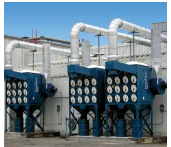
DFO on Metallizing Powder Flame 20,500 cfm (34,822 m 3 /h)
