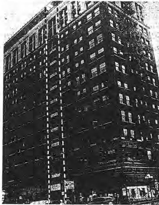
The thirteen-story, height-limit Commercial Exchange Building at Eighth and Olive streets is being sliced in half to conform to the setback line of Olive street. Superimposed dotted lines indicate the ten-foot section which is being removed.
