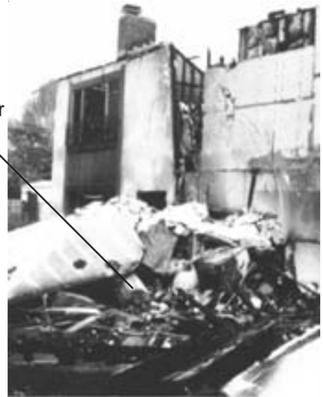
Figure 10 - The unbraced water heater in this building fell during an earthquake; the resulting fire destroyed the building.
