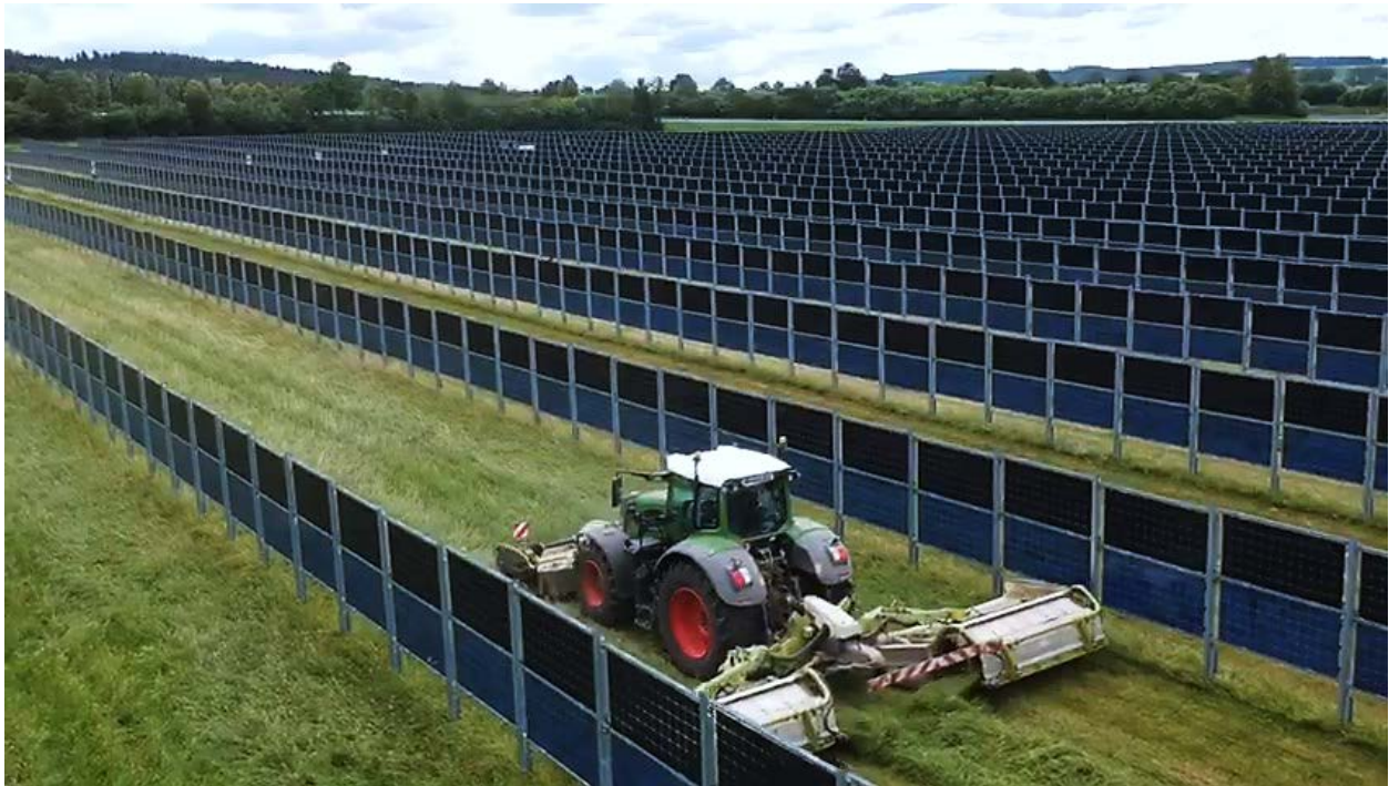
Figure S-8: Bifacial vertically-installed solar panels: Solar Farm, Donaueschingen, Germany Photo credit: Next2Sun GmbH, Germany, with permission
