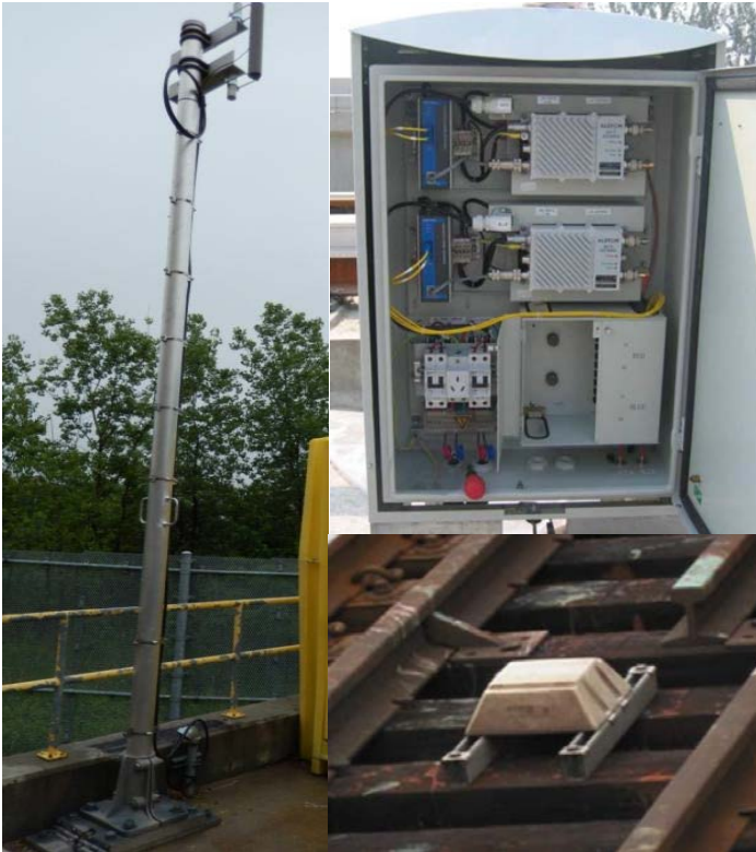
Radio Communications Equipment
