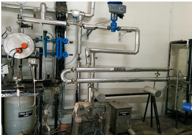
Figure: Boiler and Heat Exchanger Pilot plant
