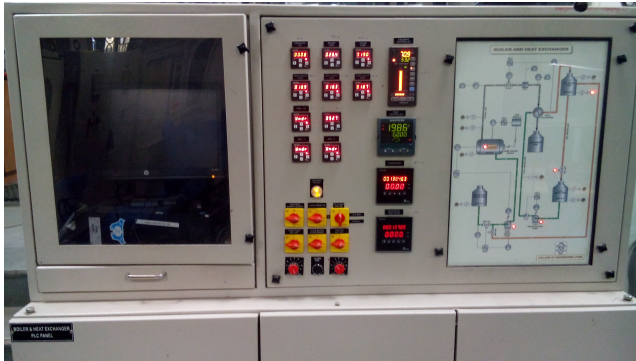
Figure: Control Room for Boiler and Heat Exchanger Plant
