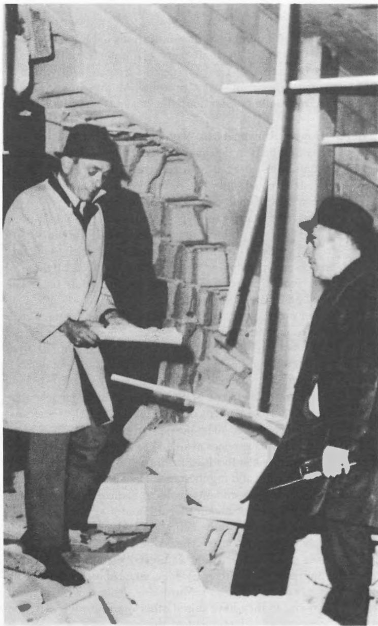
President Wendell G. Hardway (left) of Bluefield State College, West Virginia, examines bomb damage to the college's physical education building.
