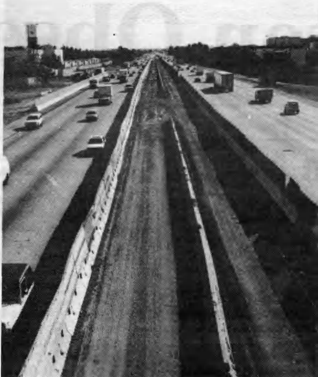
Construction of carpool lanes on the 57 freeway is underway. The project is financed by Measure M.
