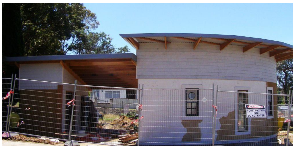
Straw bale building being constructed at Carss Park Community Garden in Sydney
