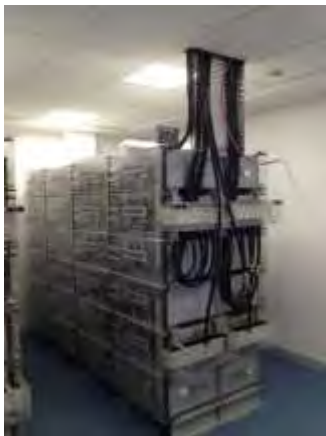
Completed battery bank
