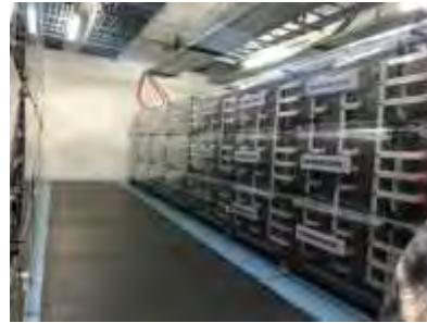
New Battery Room
