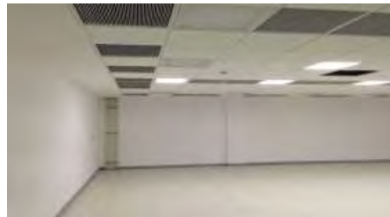
Main floor area with usage of Armstrong false ceiling, Metro Grid flooring , Promatec fire rated partitions & cable trays above and below false ceiling by legrand
