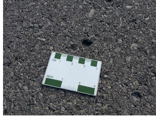
Ravelling and aggregate loss (RR 3, Haldimand County)
