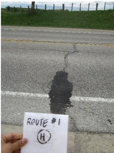
Severe damage repairs (possible potholes)
