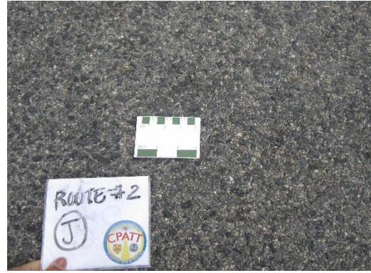
Some Aggregate loss
