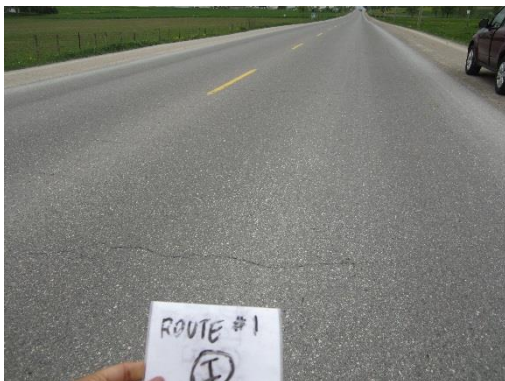
Some Thermal cracking
