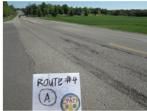
Severe wheel path damage (near an entrance; thus, slow moving traffic)
