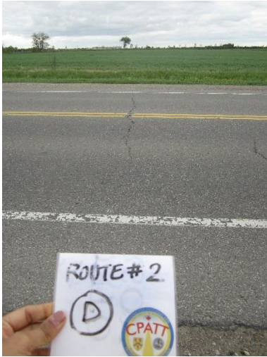
Thermal cracking in the middle of the road
