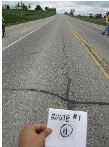
Combination of transverse and wheel path cracking
