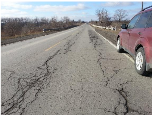
Severe wheel path rutting and cracking (RR 3, Haldimand County)
