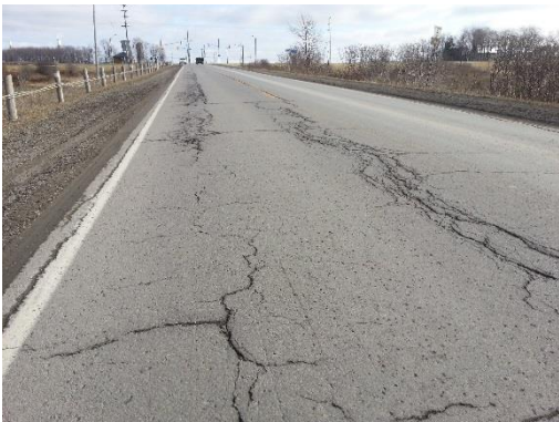
Severe wheel path cracking (RR 3, Haldimand County)
