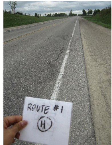
Wheel path cracking on just one side (poor to no drainage)
