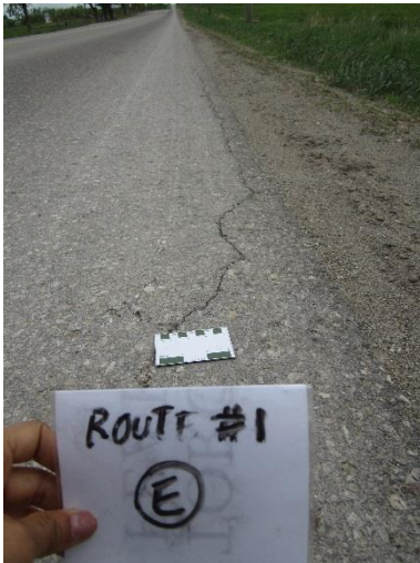
Cracking near the shoulders (poor drainage)
