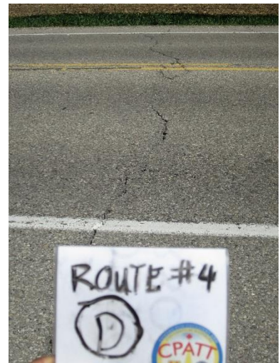
Thermal transverse cracking
