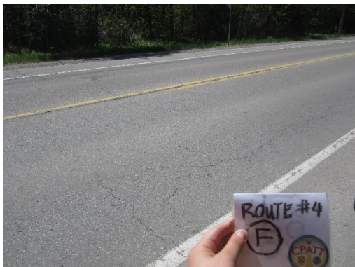
Combination of thermal and wheel path micro cracking
