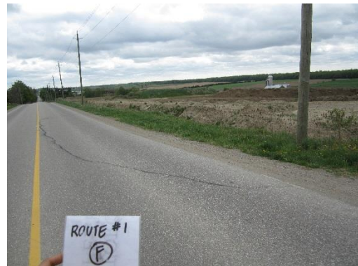
Structural damage due to poor drainage
