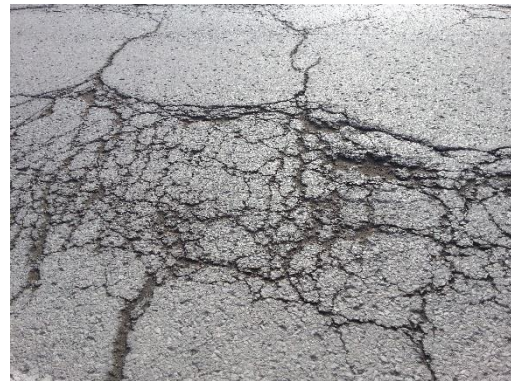
Severe alligator cracking (RR 3, Haldimand County)
