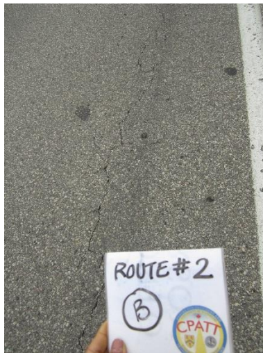
Micro cracking on wheel path
