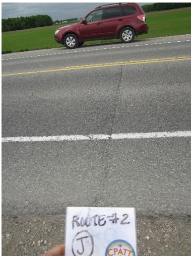
Construction joint cracking
