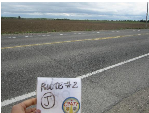
Crack at construction joints
