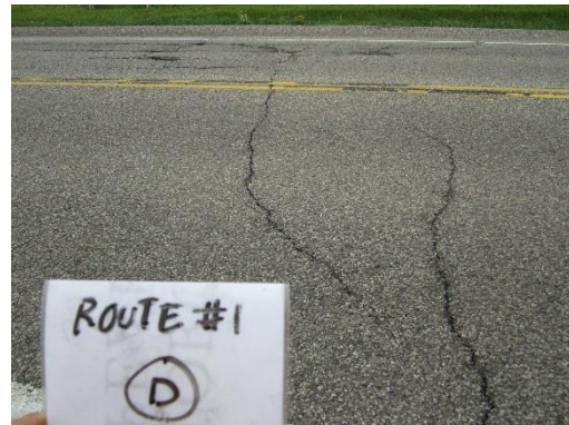
Severe Thermal transverse cracking
