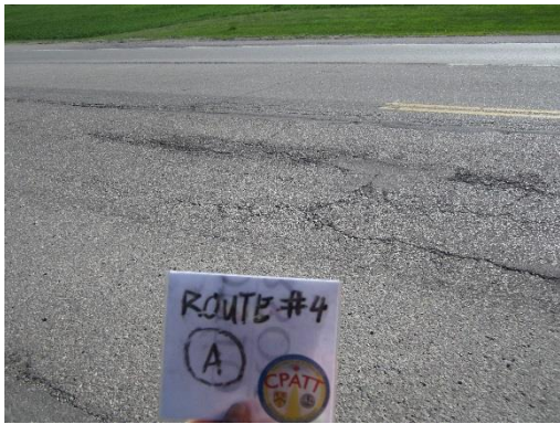
Severe cracking and possible structural damage (poor drainage)
