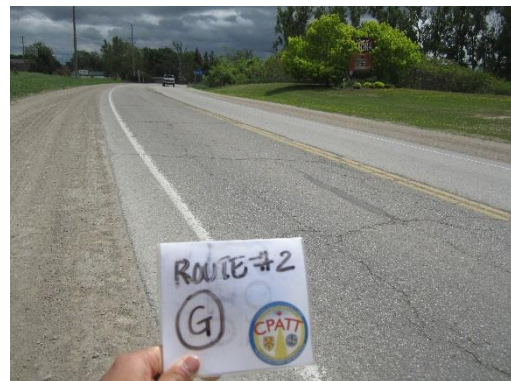
Wheel path cracking
