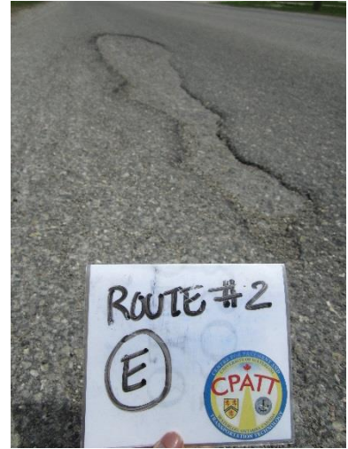
Large severe pothole and aggregate loss
