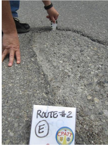
Large severe pothole and aggregate loss
