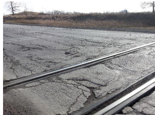
Severe cracking near railway tracks (RR 3, Haldimand County)
