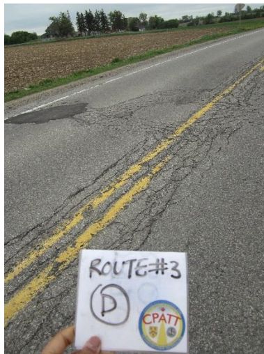
Severe alligator cracking near the centreline
