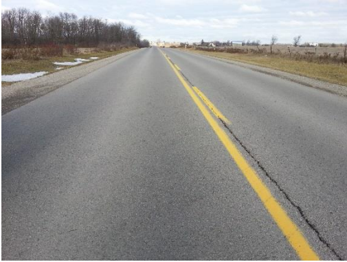
Centreline cracking (RR 3, Haldimand County)
