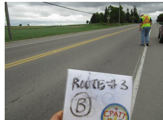
Some wheel path rutting
