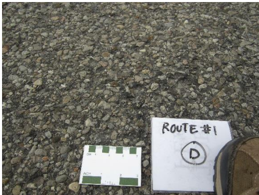
Ravelling/ Aggregate Loss
