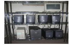
Your servers, your datacenter
