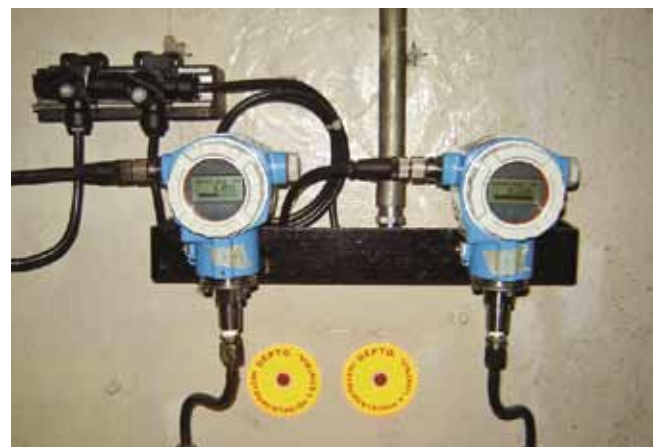
Pressure devices to monitor lube oil pressure as well as the air pressure for the air-pressurized lube oil tank. CFE CH Malpaso
